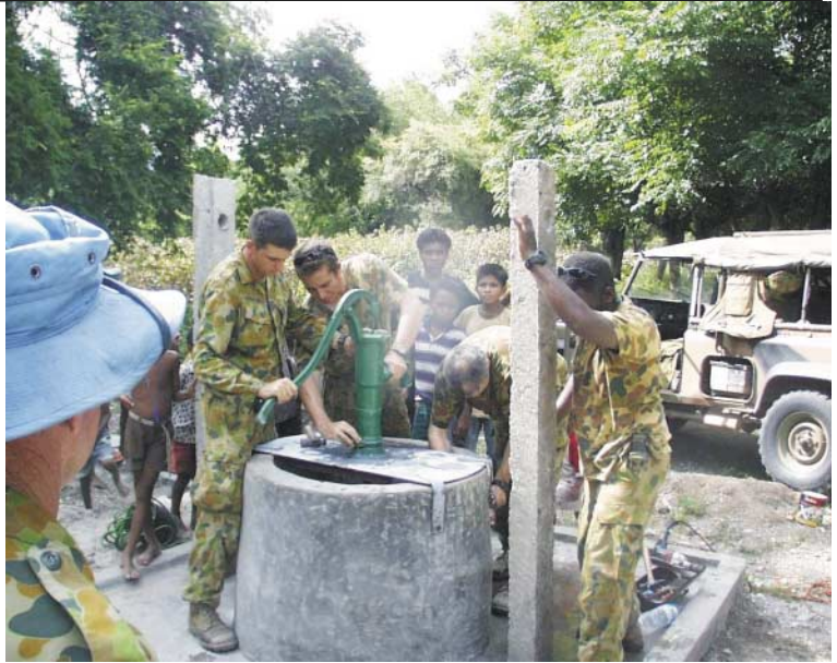
CMA Field Team (Golf 21) begin construction of the water hand pump as part of a Quick Impact Project (Hearts and Minds) at Palaka Primary School, Bobonaro District
